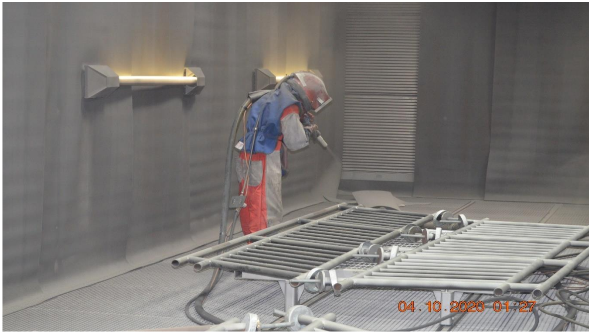
GRIT BLASTING BOOTH WITH RECOVERY SYSTEM
