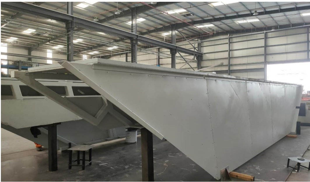
MILD STEEL FRAME FOR GLASS CLADDING
